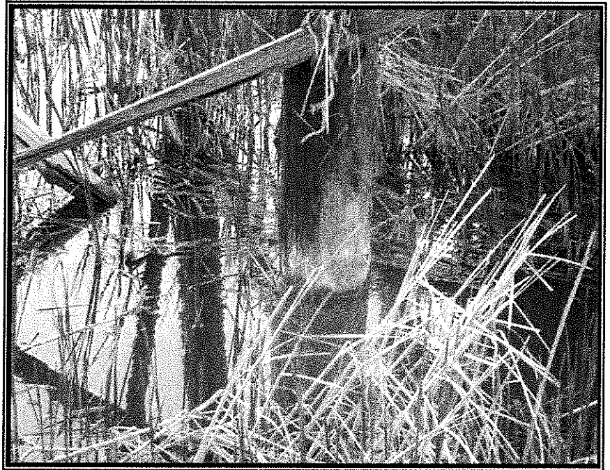
Typical Decay of Piles at Waterline - Bents 4 and 5
