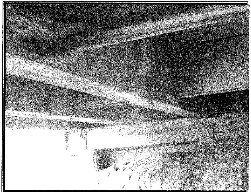
Check Crack in G3 - Span 10
