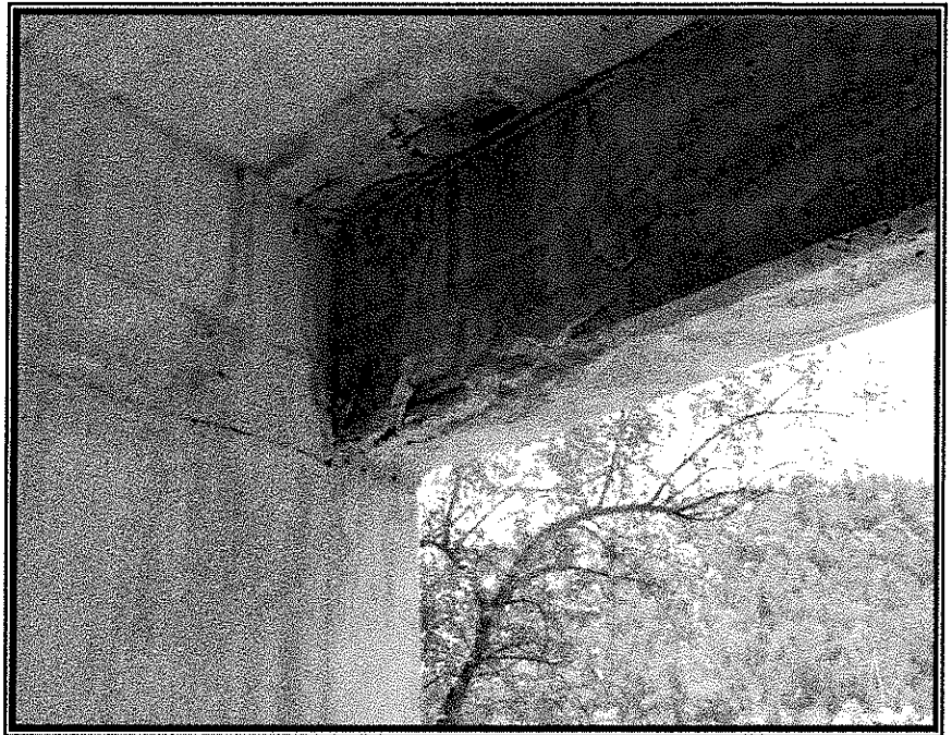
Spalling with Exposed Rebar - Beam 5 over Abutment
