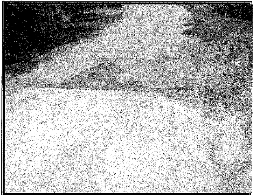
Bump Onto Bridge at West End
