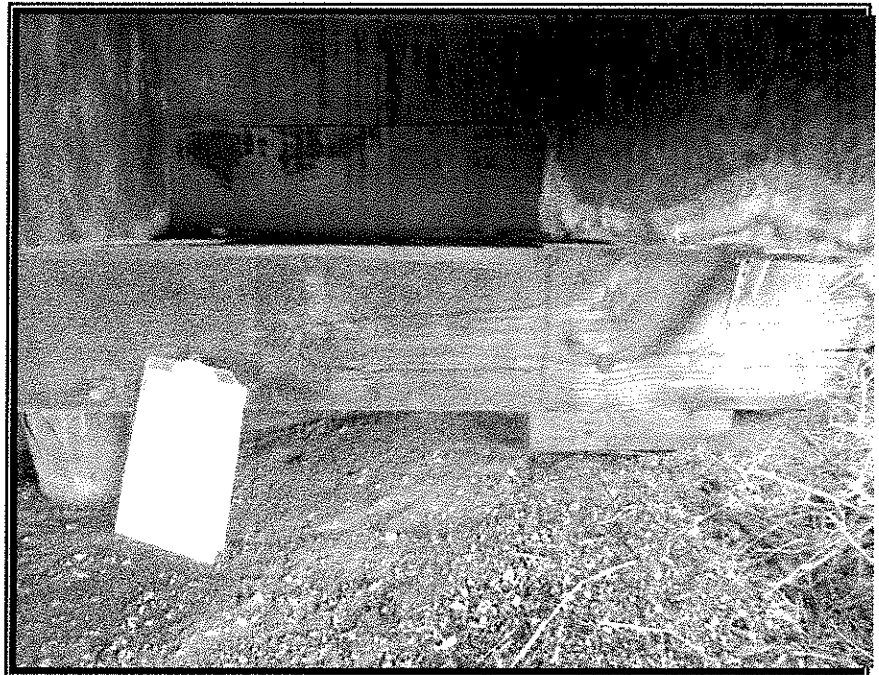
Decayed North End of West Abutment Cap
